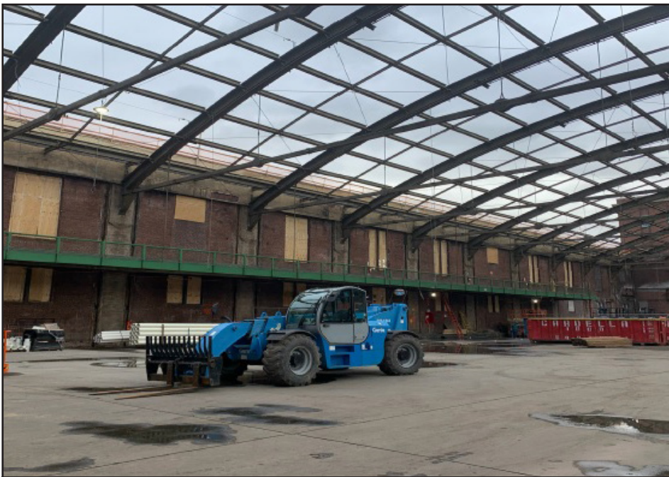
A view of the ongoing work at the Jamaica Armory Oct. 27, 2021 shows the continuing renovations to the expansive finished drill floor, with 55 feet to the top of steel and is approximately 50,000 square feet. The renovations are part of a $120 million, three-year project.
