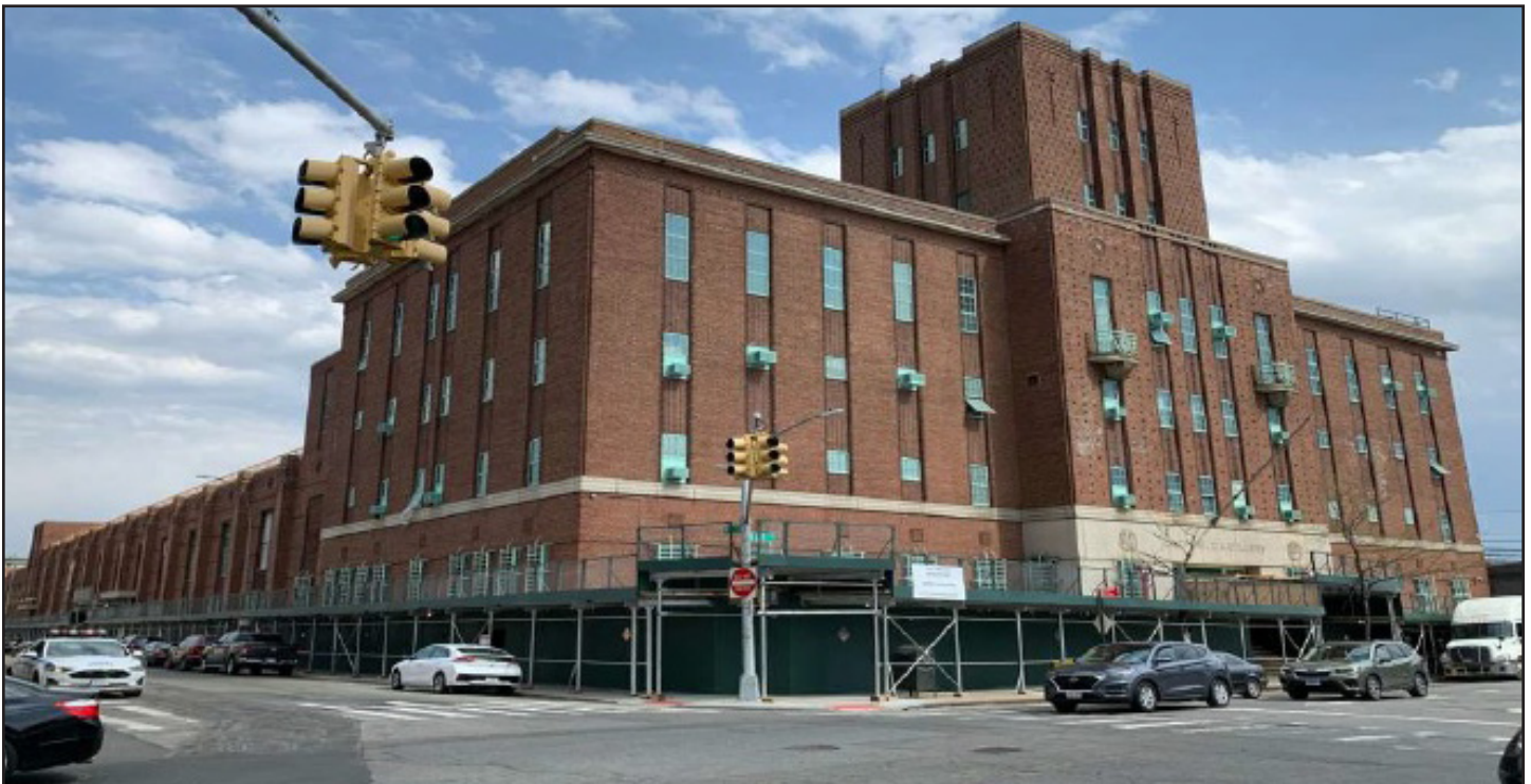
Renovations for the Jamaica Armory in Queens, New York began in 2021 with a three-year, $85.2 million contract to renovate the 140,787 square foot facility. The armory is home to the headquarters of the 1st Battalion, 258th Field Artillery.
