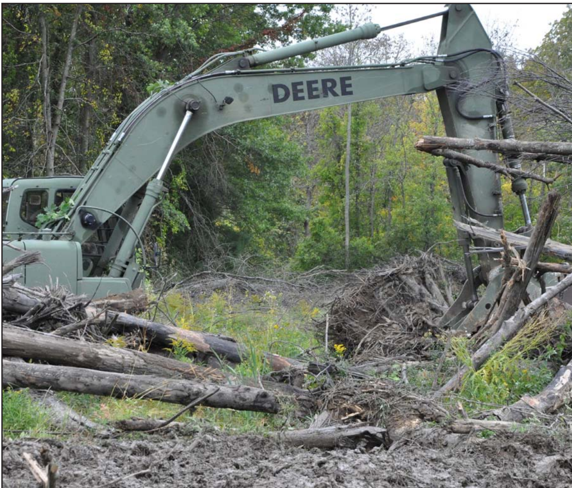
Soldiers assigned to the New York Army National Guard's 204th Engineer Battalion work to clear dead trees near Normanskill Creek in Albany N.Y. on Oct. 2, 2015 as part of preparations for the possible landfall of Hurricane Joaquin. At the direction of Gov. Andrew M. Cuomo members of the battalion were mobilized to work with the New York State Department of Environmental Conservation to clear obstructions from waterways which could cause flooding during a heavy rainfall. As part of the process, the engineers created space where debris from the stream could be deposited.
