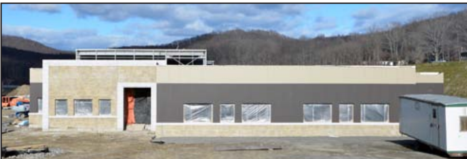
Construction of the new Combined Support Maintenance Shop at Camp Smith Training Site continues. The new facility, due to be completed in 2017, will provide support to units on Long Island and in New York City and the Hudson Valley.
