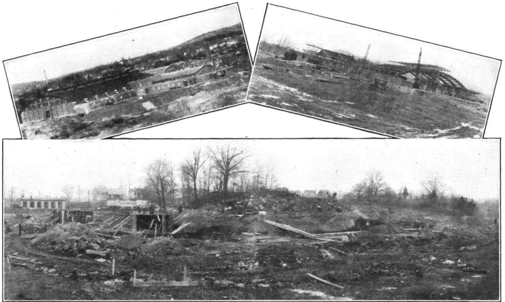
These three photographs, all taken on the same day (March 1st, 1932), show the respective stages of construction of the three new armories for the 156th Field Artillery at Newburgh (top left), Kingston (top right), and at Peekskill, N. Y. Ground was broken on the Peekskill site on January 7th and it is hoped that the building may be ready for occupancy by November, 1932.
