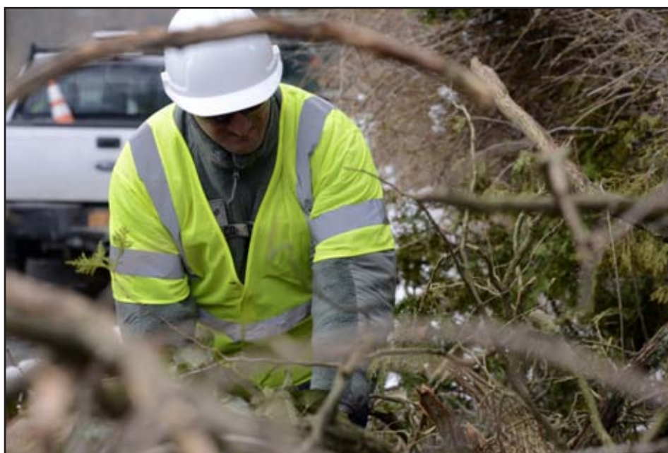
An Airmen assigned to the 105th Airlift Wing helps town and county workers clear debris from roadways in Putnam County, N.Y. deployed to Putnam County, March 7, 2018. The county was hit hard with a winter storm knocking down trees and causing widespread power outages.
