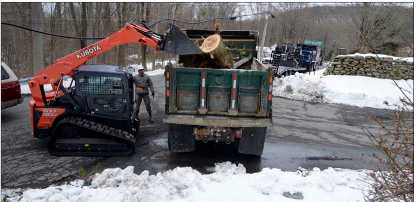
Airmen from the New York Air National Guard's 105th Airlift Wing move debris from a road in the town of Carmel, N.Y. on Monday, March 5. Twenty Airmen assigned to the 105th Airlift Wing deployed to Putnam County, New York, to help town and county workers clear debris from roadways.
